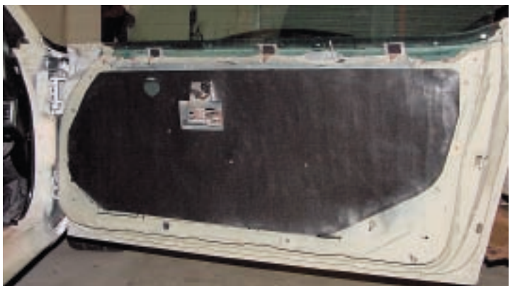
Photo #3: We then installed fresh string caulk, part #49-49 , to the back (uncoated) side of the barrier and affixed it to the inside of the door. Note the power door lock plug above the inside door handle.
